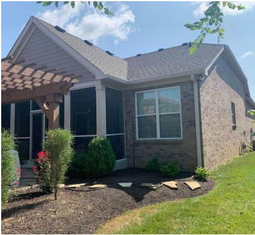
Component(s): Fascia, Siding
