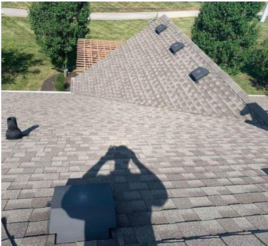
Component(s): Box Vent, Shingles Overview, Pipe Vent
